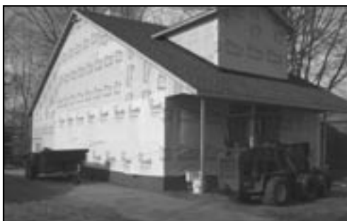
This home is being renovated and enlarged in the North end of the city.
